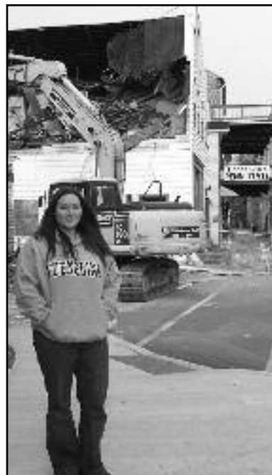
Jen Buck, manager of the Scarlet D stands in front of the demolition project of a long standing eyesore building at the corner of Chestnut and 3rd Streets. The Scarlet D purchased the corner property and will make it part of their restaurant, bar and hotel complex. ❁
